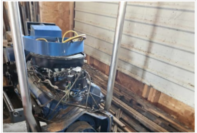
#LLA INTEK 190 PUMP UNIT
