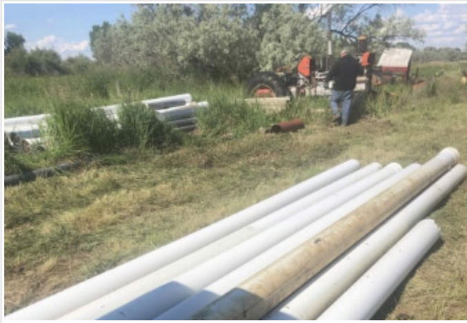
#125 8 inch PVC pipe
