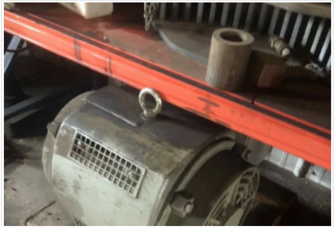
#HTK Converter Unit
