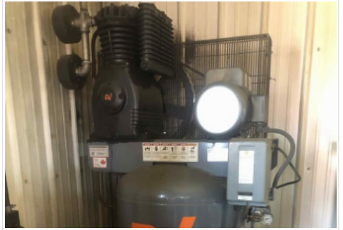
#HTK Standup Right Air Compressor
